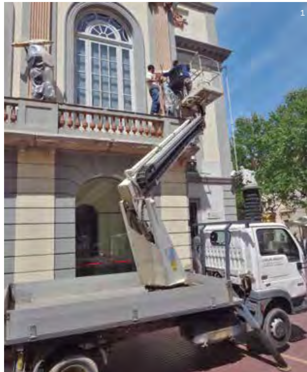
1, 2. Work on the façades of the Theatre-Museum in Figueres and the Castle in Púbol
